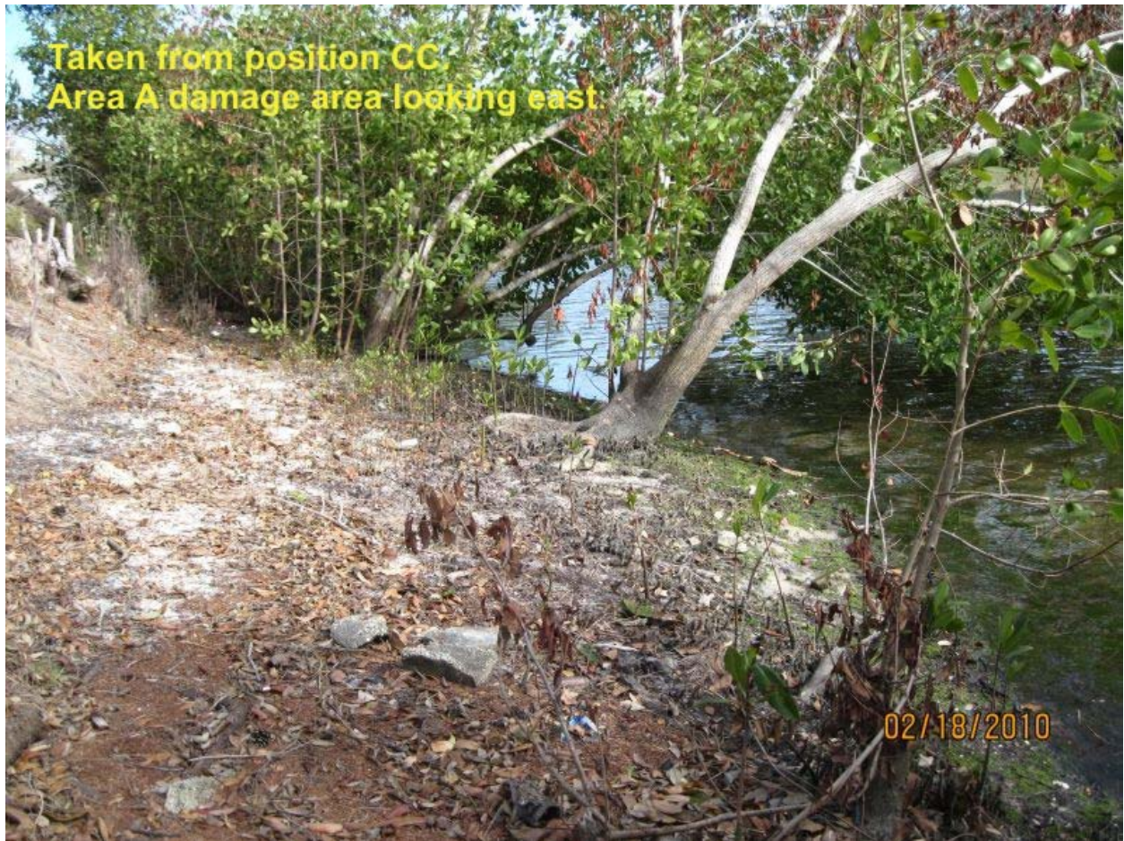
This was taken at position CC, standing just above the low tide water line, leaning against the south most Australian pine at the west end of Area B. It shows the damage area in Area A.
